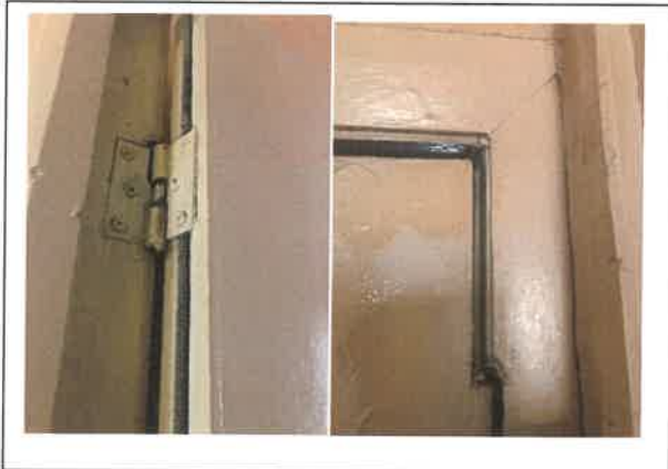
Fig 9: Flat 4 entrance door has gaps in excess of 3mm from the door to the frame and is fitted with non fire rated hinges.
