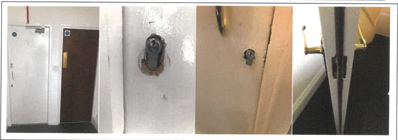
Fig 3: Unverified repairs to flat entrance doors where new locks have been fitted which in turn has compromised the integrity of the doors - recommended replacement of flat entrance doors with modern FD30s door sets
