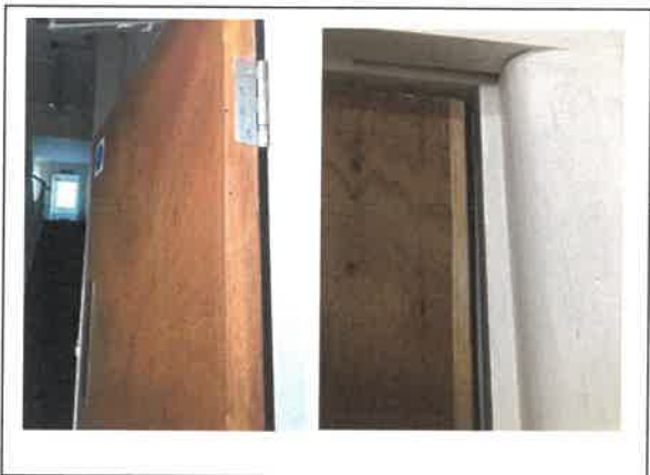
Fig 6: Gaps in excess of 3mm from the ground floor lobby door to the frame.
