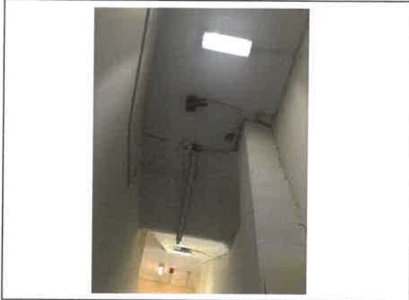
Fig 4: Heat detector at base of staircase to be replaced with smoke detector.
