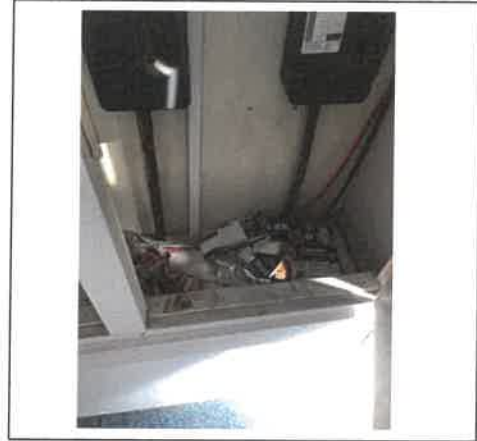
Fig 2: Waste items in base of electrical intake cupboard
