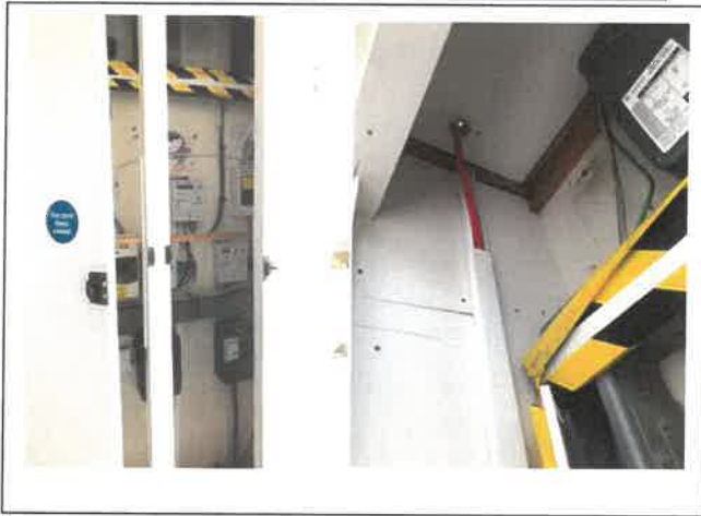
Fig 1: Non fire rated electrical cupboard (non fire rated hinges and only partial upgrade of cupboard)
