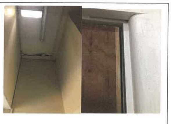
Fig 7: Poor siting of smoke detector on second floor - detectors should not be within 500mm of the wall.
