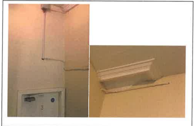
Fig 10: Fire stopping issues from flats to the common areas where alarm cables penetrate the wall and have not been suitably sealed.
