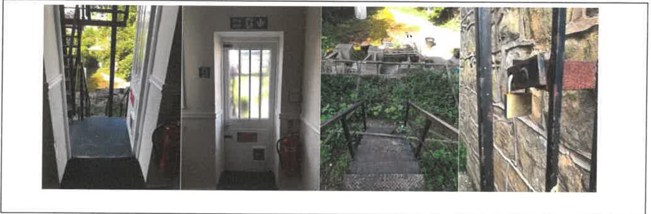
Fig 8: No easy opening devices fitted to exit doors onto external escape stair, escape stair does not discharge to place of safety due to allotment and fence at its base. Final exit gate to side of building also seen to be padlocked.
