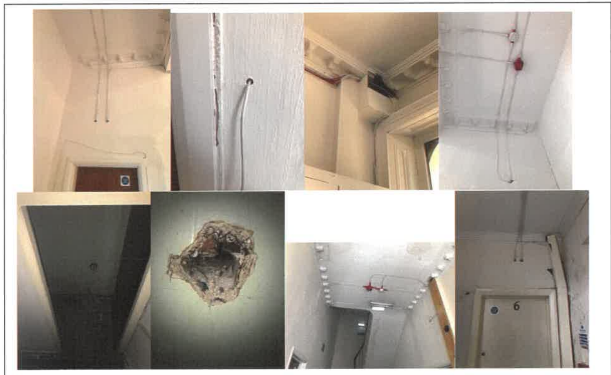
Fig 6: Fire stopping issues throughout where electrical / alarm cables have not been sealed at penetrations between floors and into flats. Further fire stopping issue noted in lower ground store at base of staircase.
