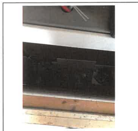
Fig 2: Small amount of waste items in base of electrical intake cupboard
