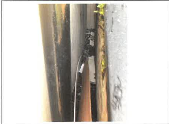
Fig 4: Build up of combustibles to side of external concrete staircase to main entrance door.
