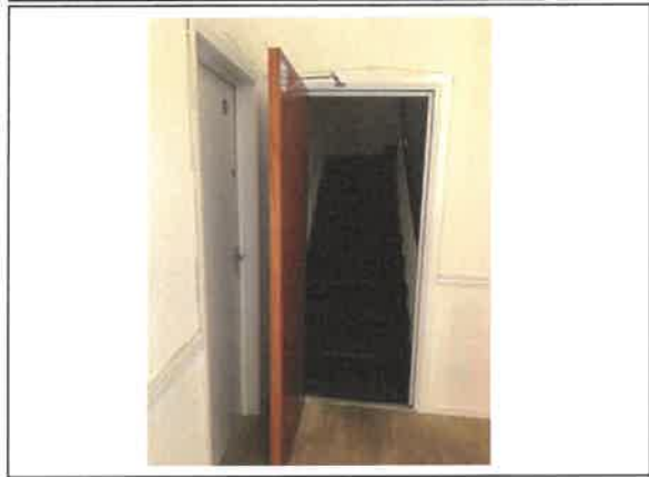
Fig 5: Ground floor lobby door not self-closing due to it sticking on the floor and also opens towards Flat 2 - door requires re-hanging so it opens away from Flat 2.
