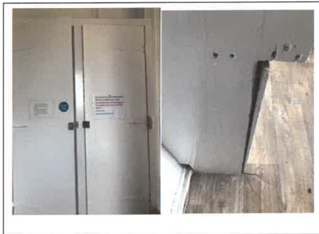
Fig 1: Non fire rated electrical cupboard (non fire rated hinges and only partial upgrade of cupboard)
